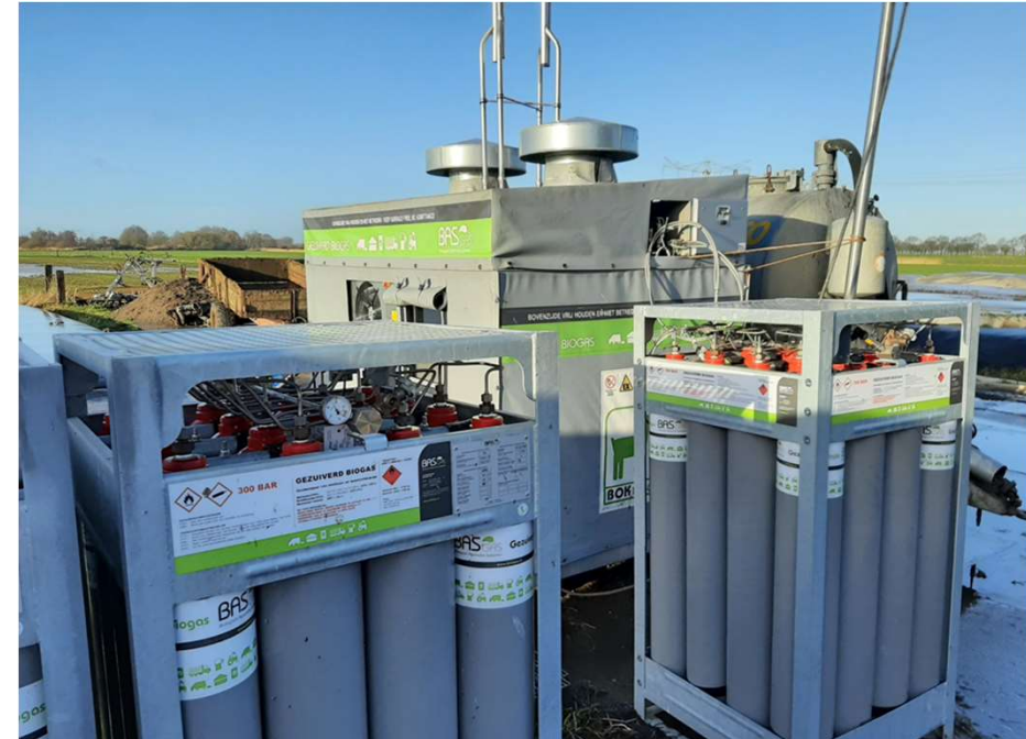
Capture, Compress Filter, Gas pipes
